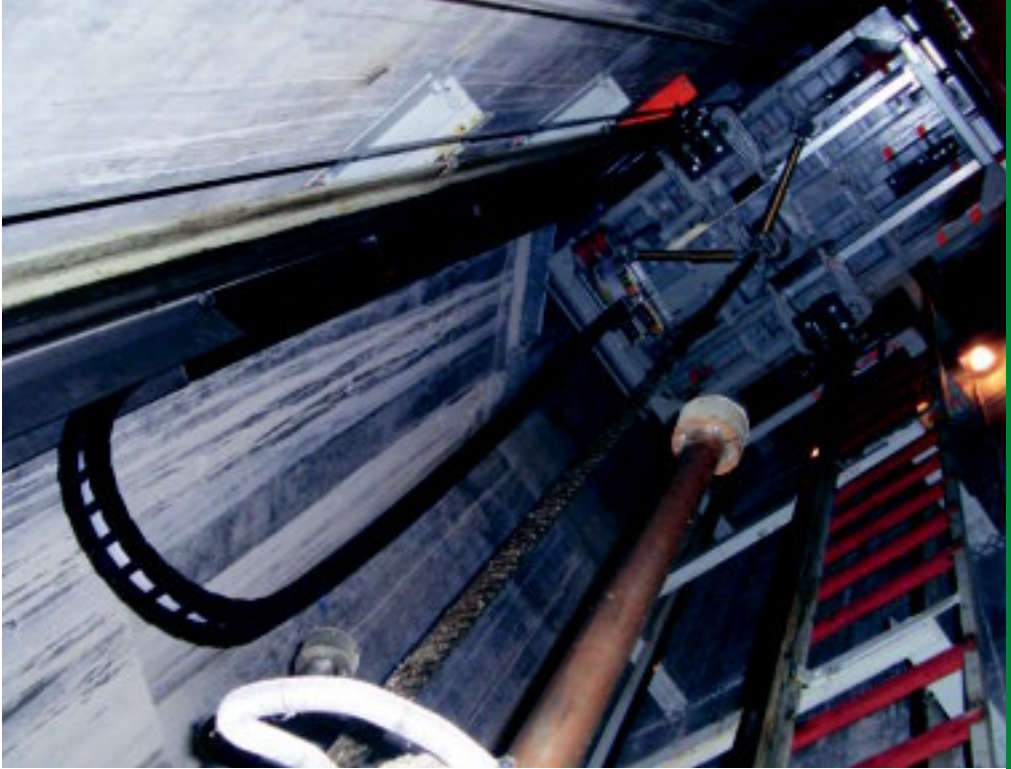
E2/000 - stability for the energy supply system elevator in a Post Tower
